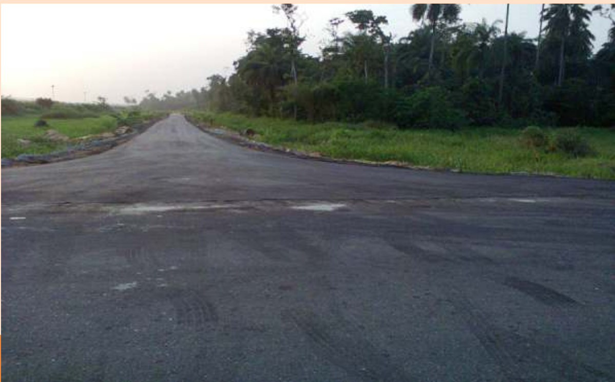
Access Road To Oilserv Manifold For Nipp Gbarain Bayelsa
