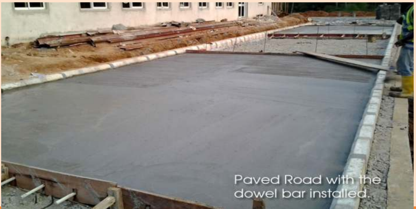
Paved Road with dowel bar at Alaoji power metering station
